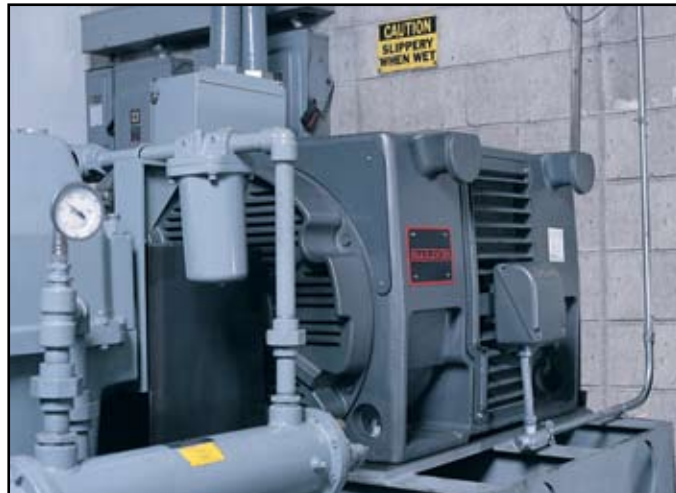
700 Hp Baldor WP11 (weather protected) motor driving a transfer pump.
